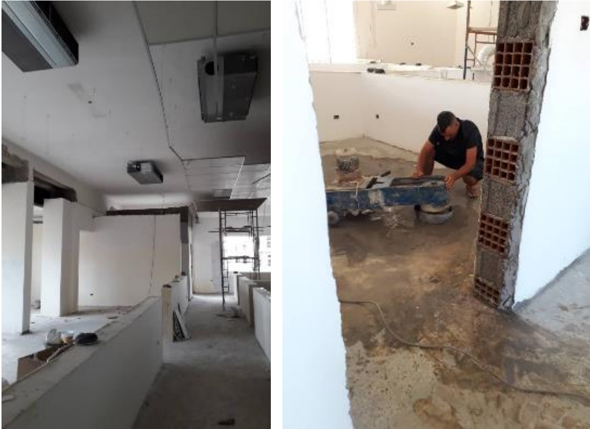
Rehabilitation works at the CCMCE offices and the handover of premises in October 2020. Photo credit: ©UNDP Libya.
